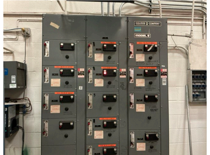
26 - MOTOR CONTROL CENTER
