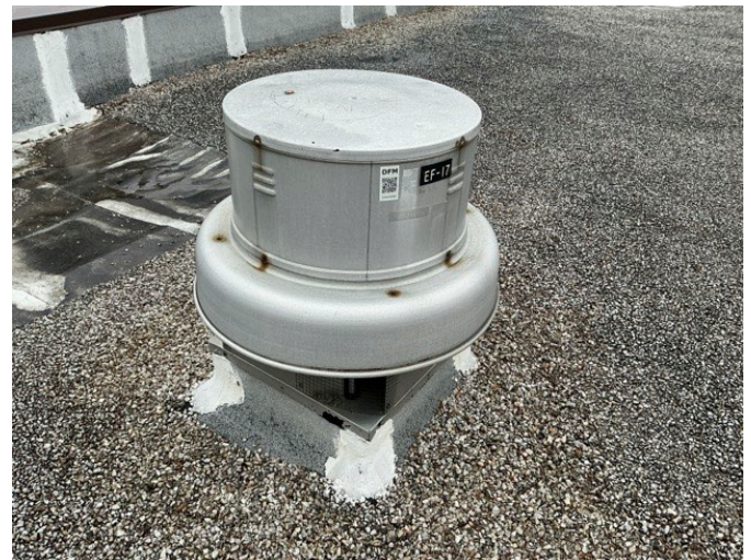
22 - TYPICAL EXHAUST FAN
