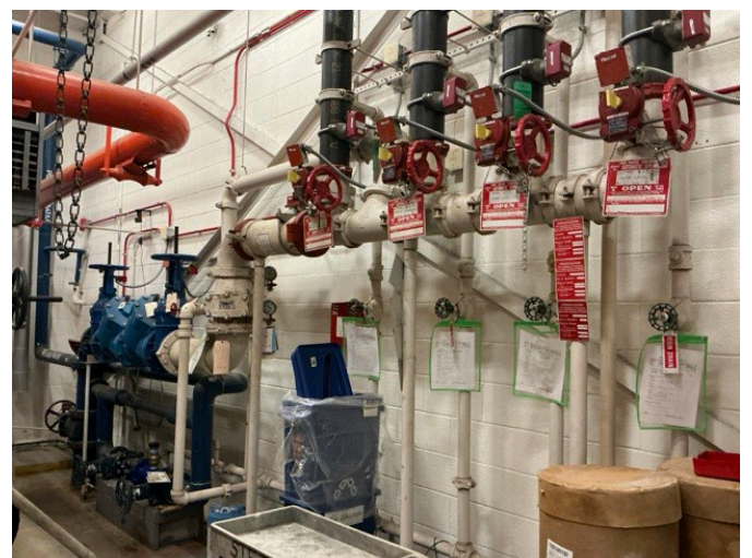
30 - FIRE SUPPRESSION SYSTEM
