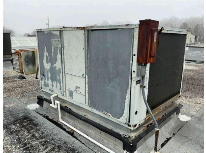
20 - TYPICAL PACKAGED UNIT
